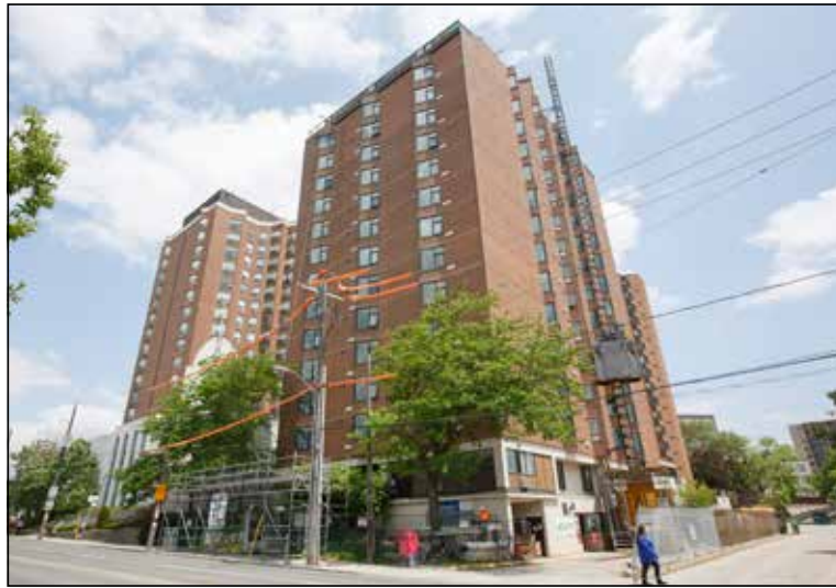
Renovations are underway at St. Hilda's Seniors Community in Toronto. The complex will include 80 apartments for previously unhoused people. PHOTO BY MICHAEL HUDSON
